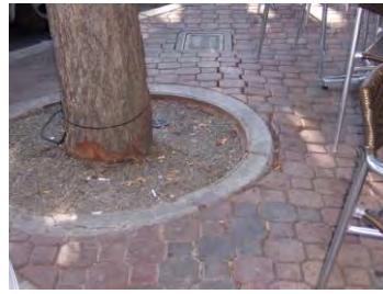
Concrete ring raised by roots Trunk is large enough the grate was replaced with DG
