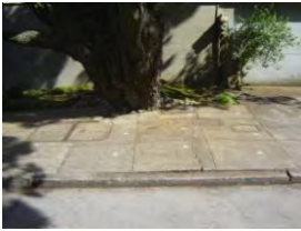
Before: Damaged sidewalk by Monterey Pine
