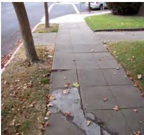
Roots raising sidewalk
