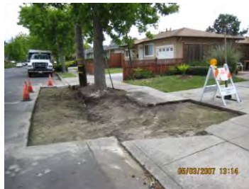
Large roots under sidewalk and driveway
